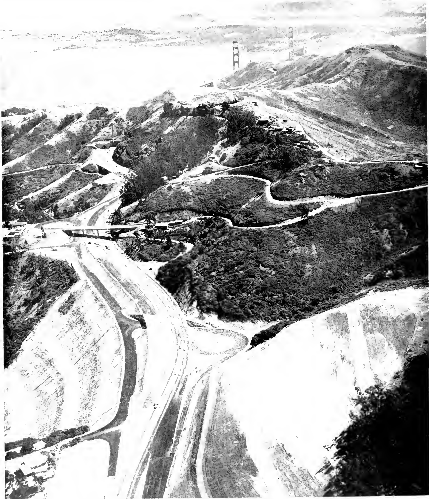
Recent aerial view of new Waldo approach to Golden Gate Bridge looking toward San Francisco. Picture graphically shows size of cuts. On September 28 both north and south bound traffic was routed through new east Waldo tunnel pending remodeling of the old bore which will require about three months.
